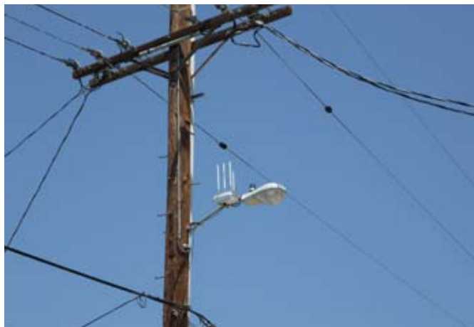
Tropos router on utility distribution pole in Glendale
